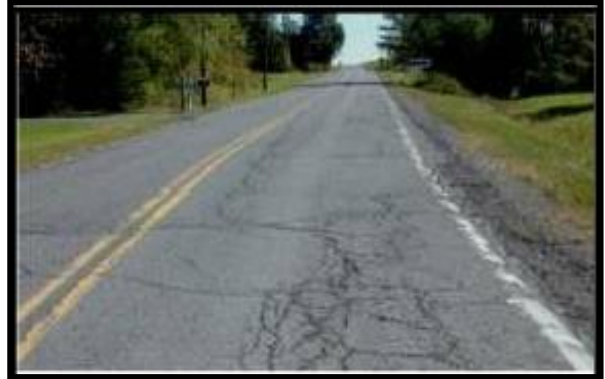
Fatigue cracking and wheel rutting.
